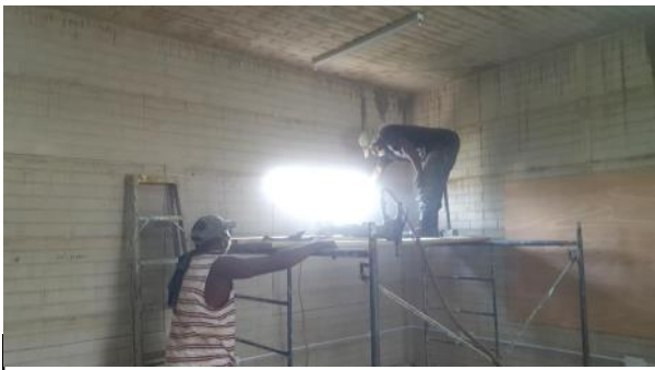
The first rays of light found their way into the new classrooms in the Belize City Friends Center. In the image, workers are cutting windows into the walls.
